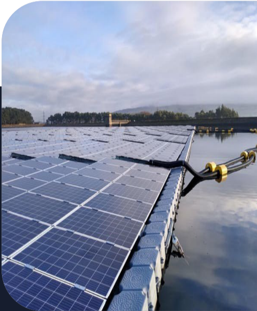
50MW + Capacity installed in Floating Solar Power
